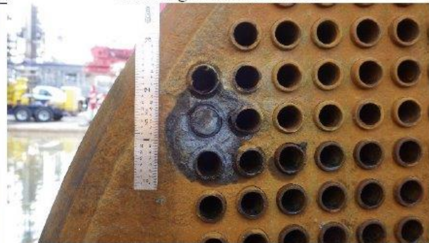
Close-up of tube/tube-sheet damage from previous photo.
