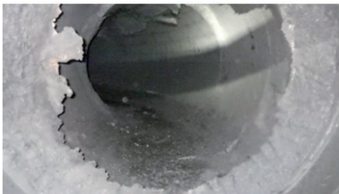
Figure 9 Fractionator inlet coke build-up
