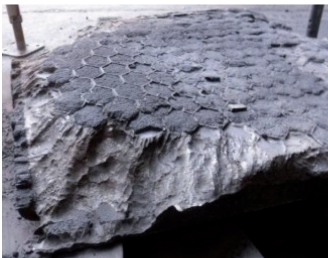
Figure 2 Severely eroded slide valve gate
