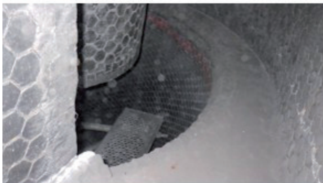
Figure 5 Primary cyclone inlet refractory damage
