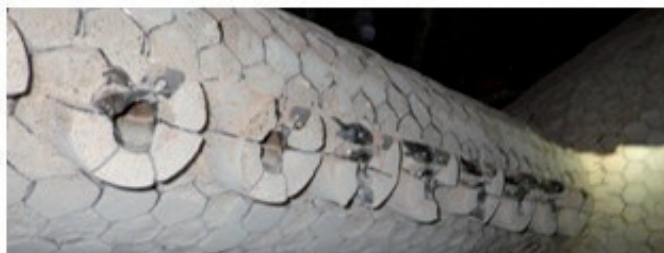
Figure 1 Air distributor nozzle erosion
