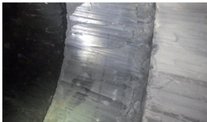
Figure 8 Reactor overhead isolation valve coke build-up
