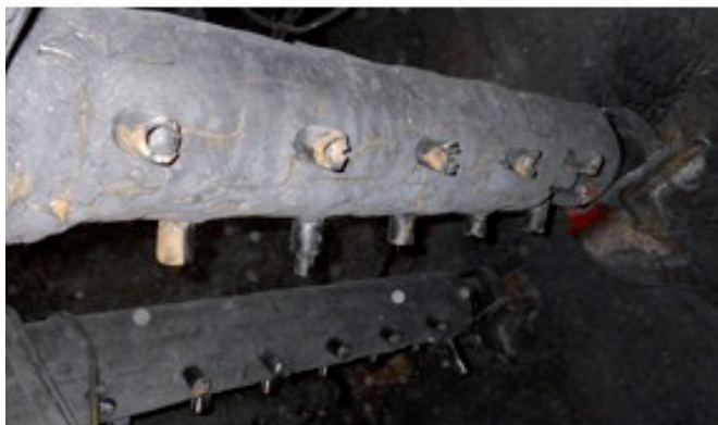
Figure 7 Steam distributor nozzle erosion
